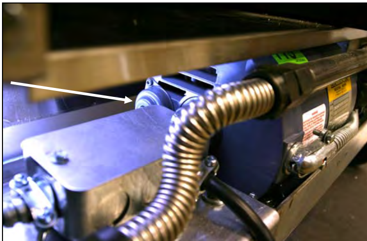
Filter Pump Reset Switch (Arrow)
